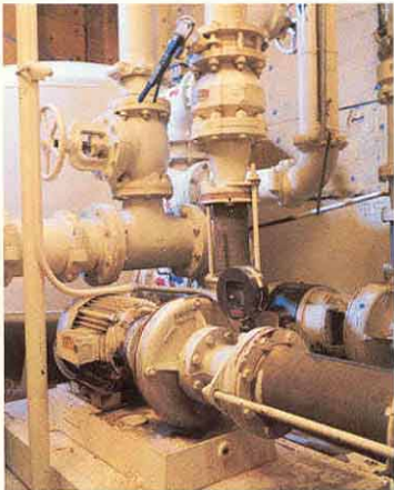
The egret fountain is operated by a 300-gallon-per-minute pump (above) that circulates water from the reflecting pool.
